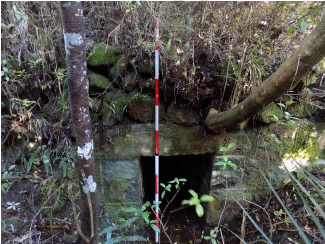
Figure 30: Culvert made from dressed stone set in mortar south of Whatoro Station.
