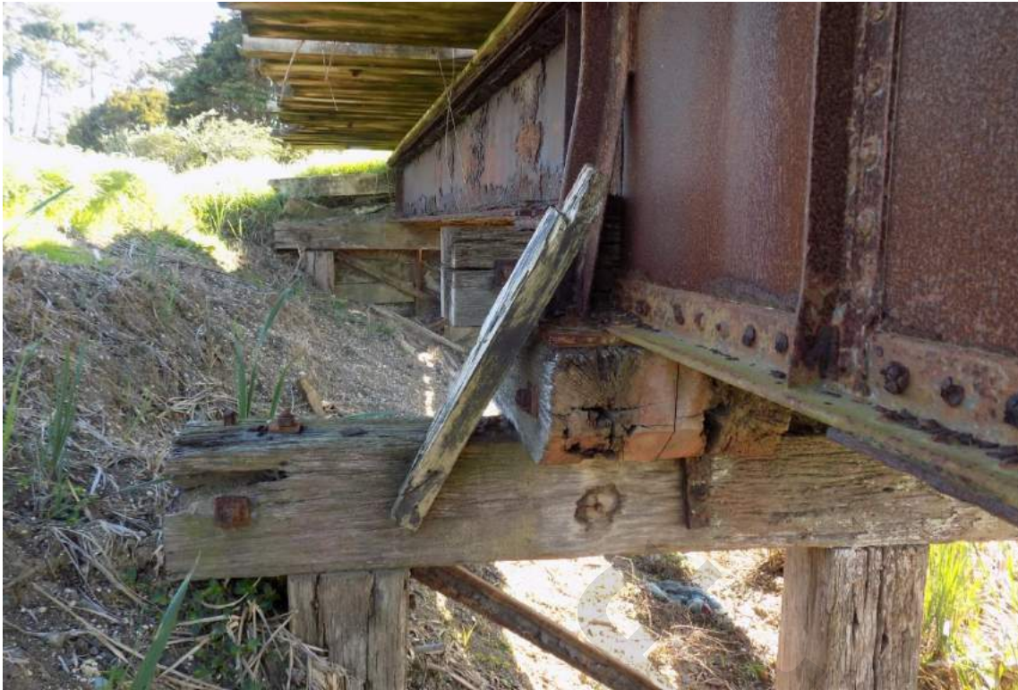
Figure 17: One of the most intact bridges surviving is between Dargaville and Parore just west of the Kaihu River. The wooden piles and bearers may be original while the iron girder is a replacement for an earlier surface. There is a farm track around the bridge to left and the bridge is no longer in use.
