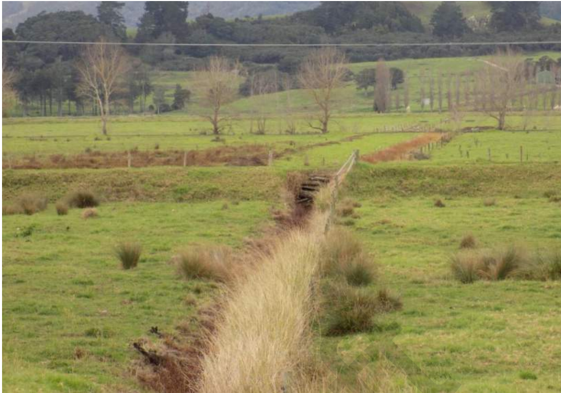
Figure 29: A culvert and drain under the railway formation between the former Maitahi Station and where the road used to cross the railway. It is visible from SH12. The track here is used as a cattle race.
