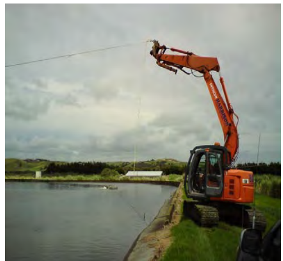
Contractors removing aerator from Dargaville oxidation pond with the assistance of a digger
