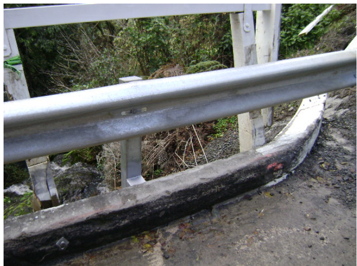
Damage to Omana Road Bridge
