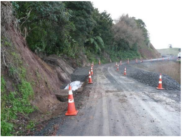
Slump partially repaired
