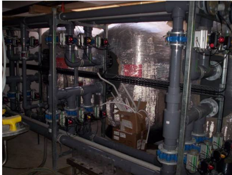
Maungaturoto Treatment Plant filters and pipework
