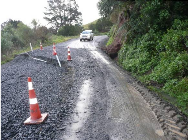
Omana Road slump
