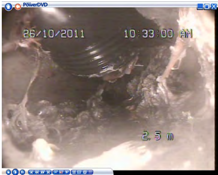
Closed circuit television footage of an illegal storm water connection made directly into a wastewater pipeline
