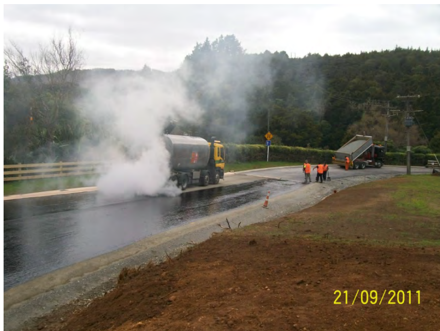
Trounson Park Road: Hot Bitumen being sprayed to form the road surface
