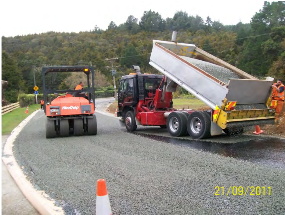
Trounson Park Road: Stones being tipped on top of the hot Bitumen and rolled in, to form the road surface.
